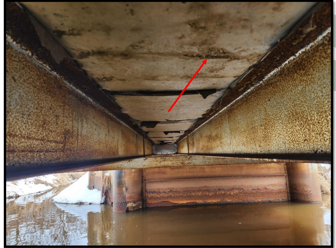
Existing conditions - spalling bridge deck
