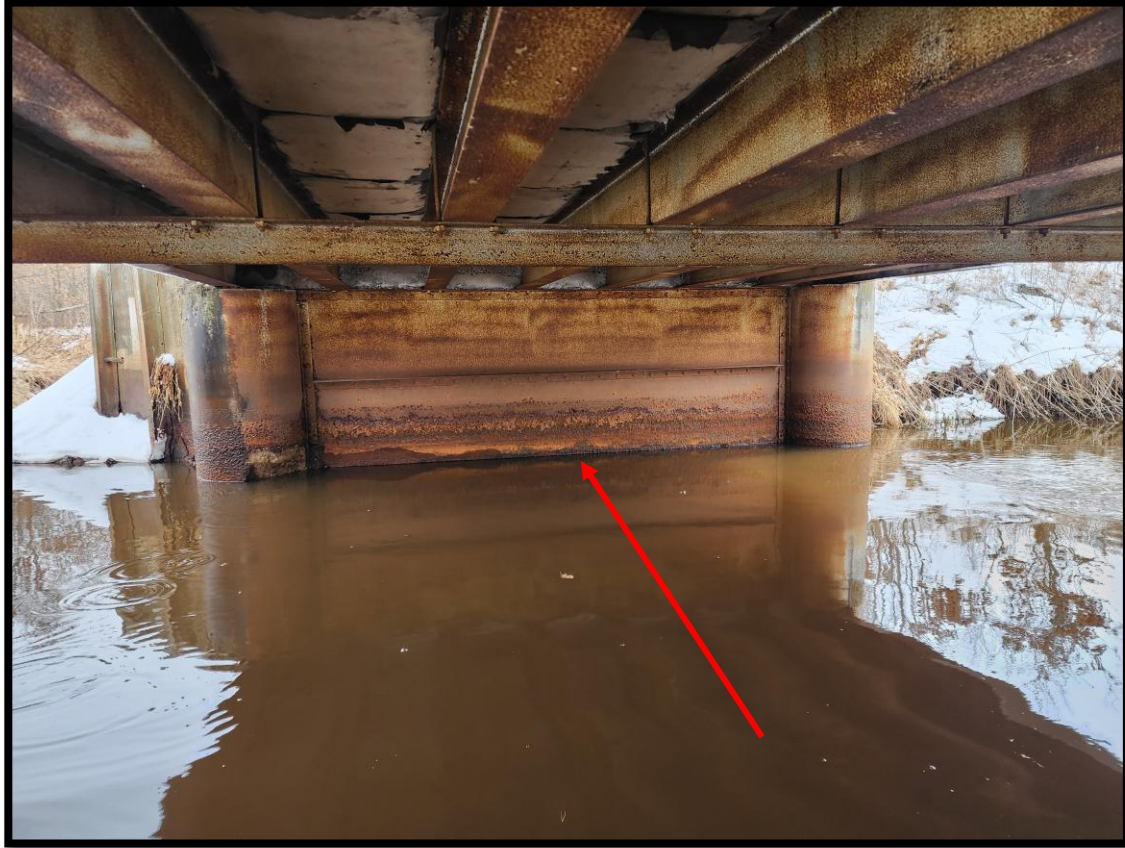
Existing conditions - section loss at waterline
