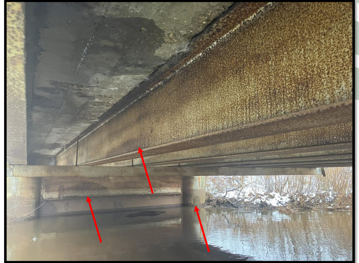
Existing conditions - columns, abutment, and girders rusting
