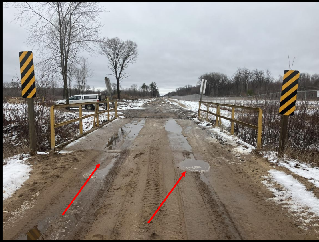
Existing conditions - approach roadway settling; ponding water
